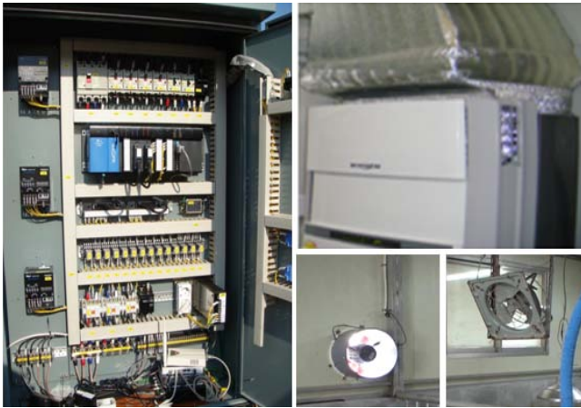
Figure 11. PLC and Livestock Farm Facilities
