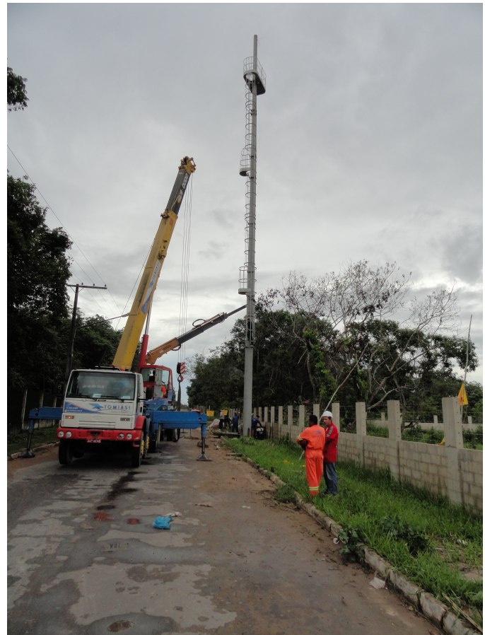
Figure 3. Pole photo installed in the Macurani Road
