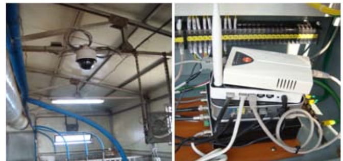
Figure 10. CCTV and DVR
