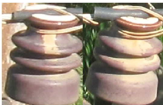
Fig. 2. Insulators presenting soot deposited on the surface
