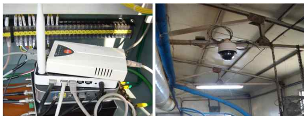
Figure 12. DVI and CCTV
