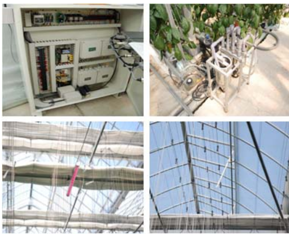
Figure 10. Greenhouse Facilities and Power Controller
