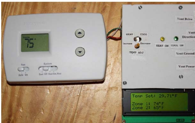
Figure 10. Integrated HVAC Control Module
